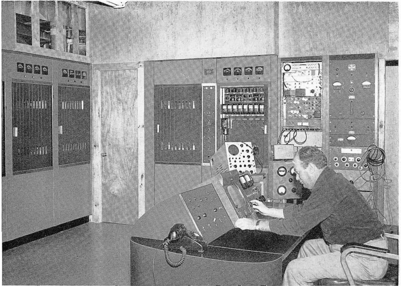
FIG. 5. Jesse H. Gibson, Transmitter Engineer, at the TTC-1B Transmitter Control Console. Control panel immediately to his right provides remote control of diesel generator power plant in the basement.
